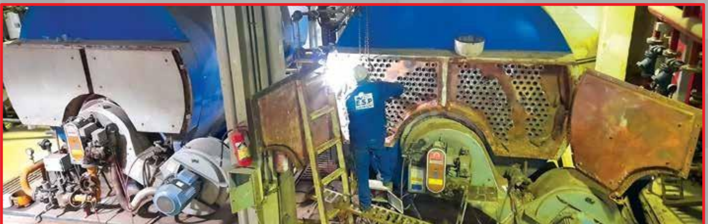
Retube MSA Boiler
