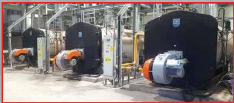
ICI Boiler and Baltur Burner
