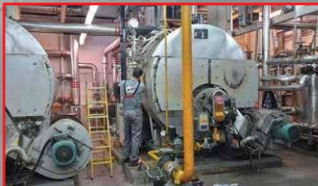
MSA Boiler Service
