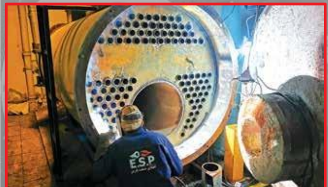
Boiler Base Plate
