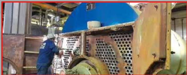
Retube MSA Boiler
