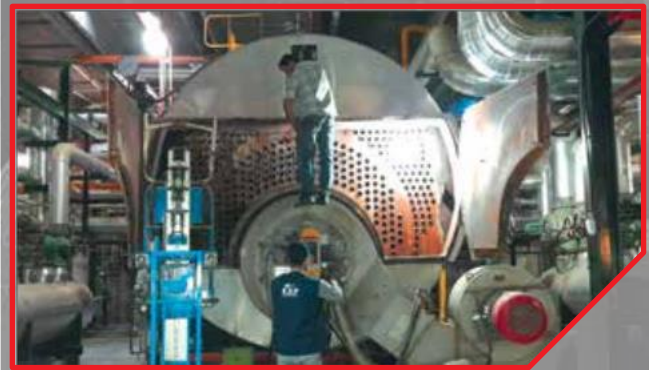
Retube MSA Boiler
