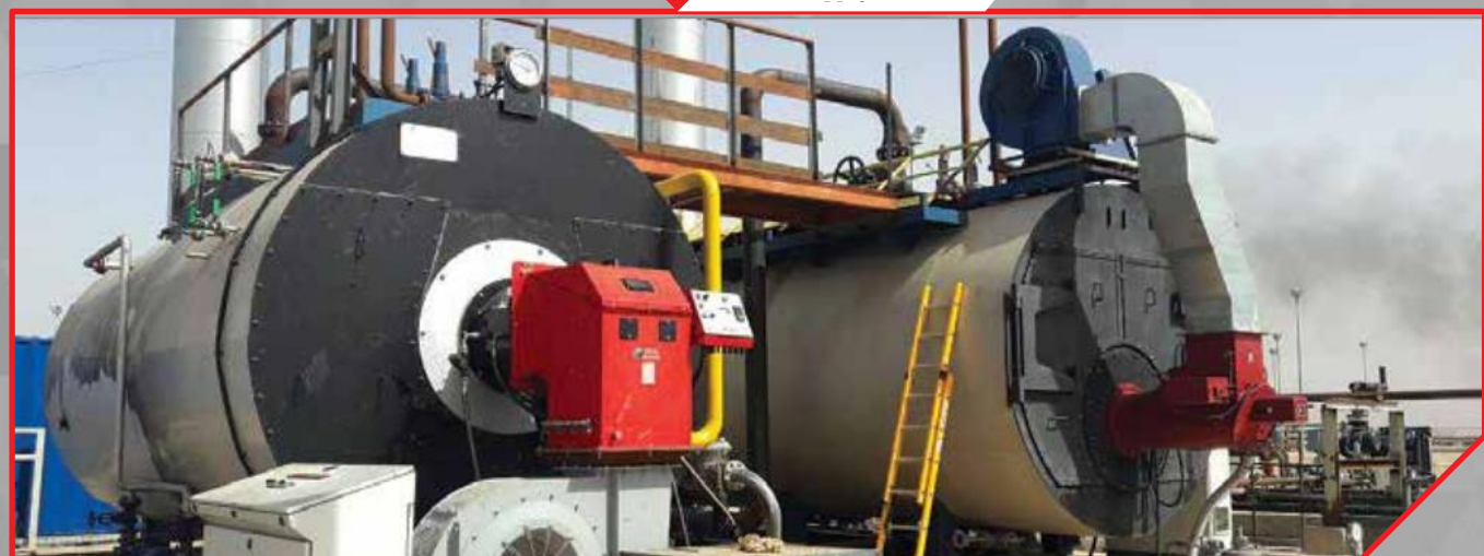
Italy Boiler and Burner Maintenance
