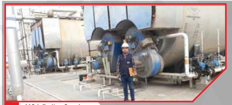
MSA Boiler Service
