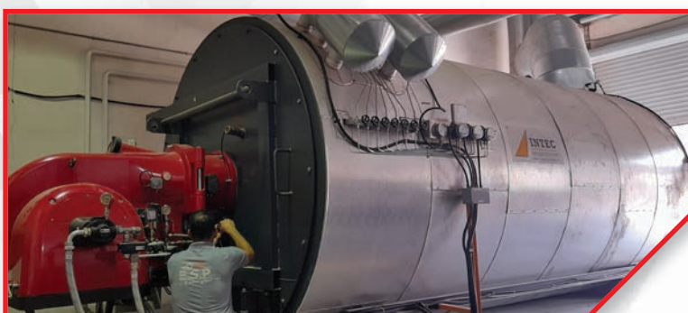
MSA Boiler Service
