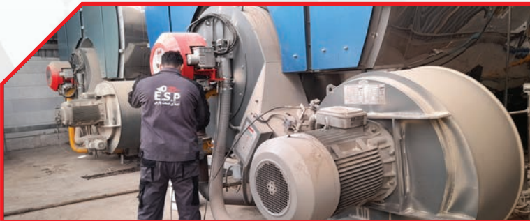
Hamworthy Burner Adjusting
