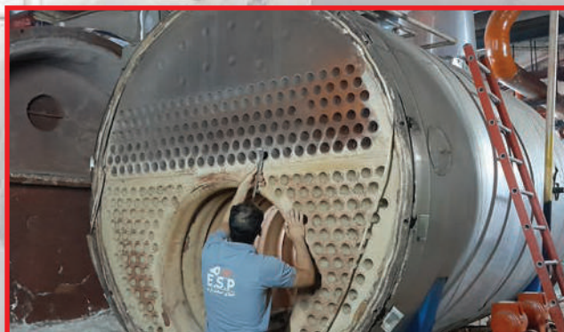
Cleaver Brooks Boiler Maintenance
