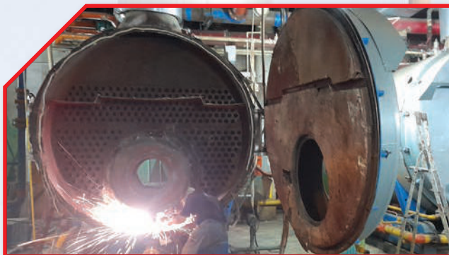
Cleaver Brooks Boiler Maintenance
